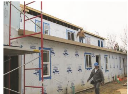
The last row of two-story homes is under construction at the Poplar Grove development site in SW Longmont.
